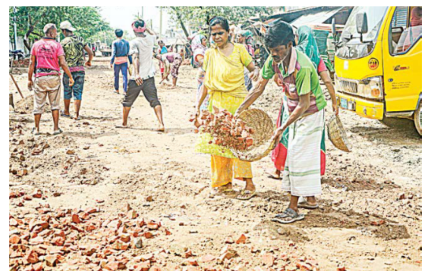
Locals have been urging the authorities to fix the MA Bari Link Road near Sonadanga Bus Stand in Khulna for 10 years but to no avail. However, they have decided not to depend on the authorities anymore and started repairing the road on their own. This photo was taken recently.
