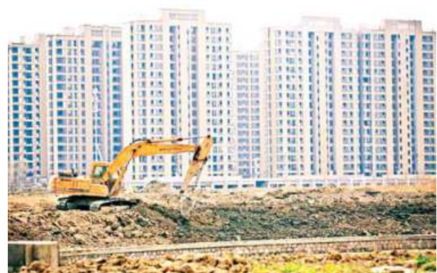
An excavator is seen at a construction site of new residential buildings in Shanghai, China.
