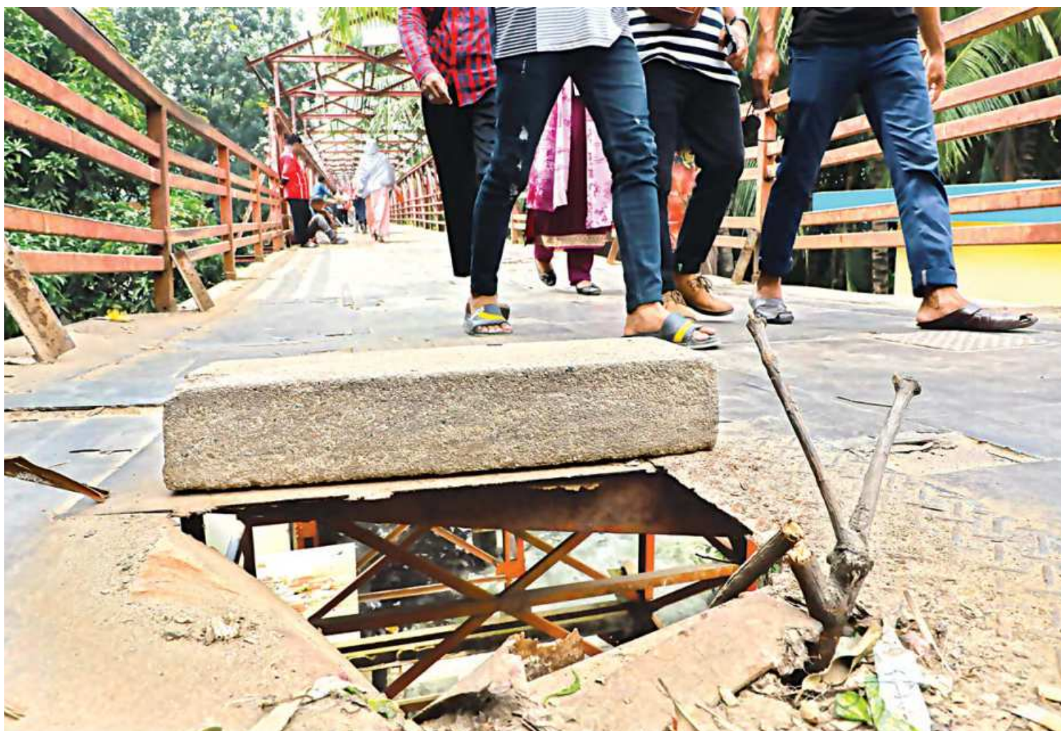
A lack of maintenance caused such severe damages to the foot overbridge right in front of the gate of Kamalapur Railway Station, causing accidents on a regular basis, say locals. The photo was taken yesterday.
