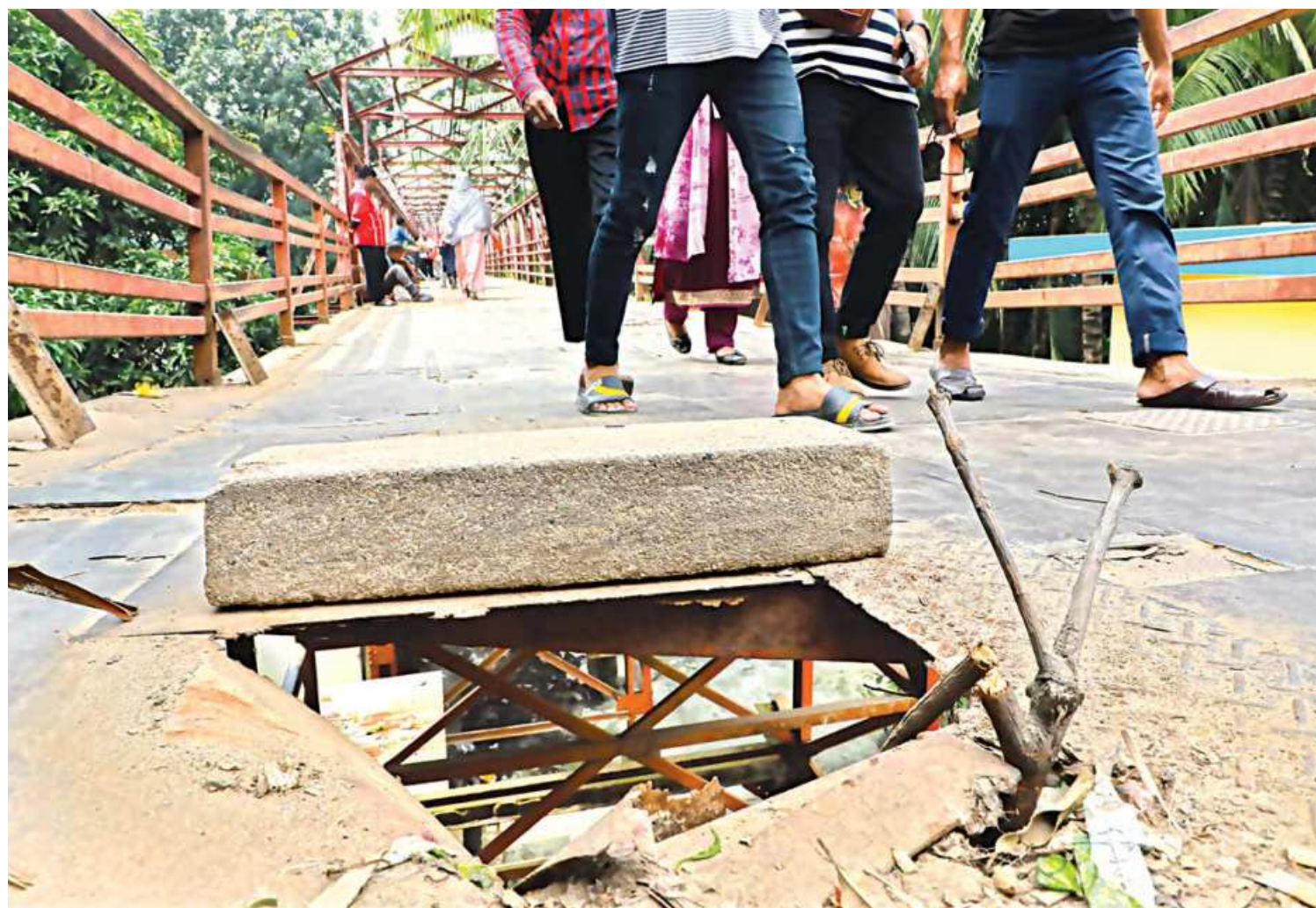
A lack of maintenance caused such severe damages to the foot overbridge right in front of the gate of Kamalapur Railway Station, causing accidents on a regular basis, say locals. The photo was taken yesterday.
