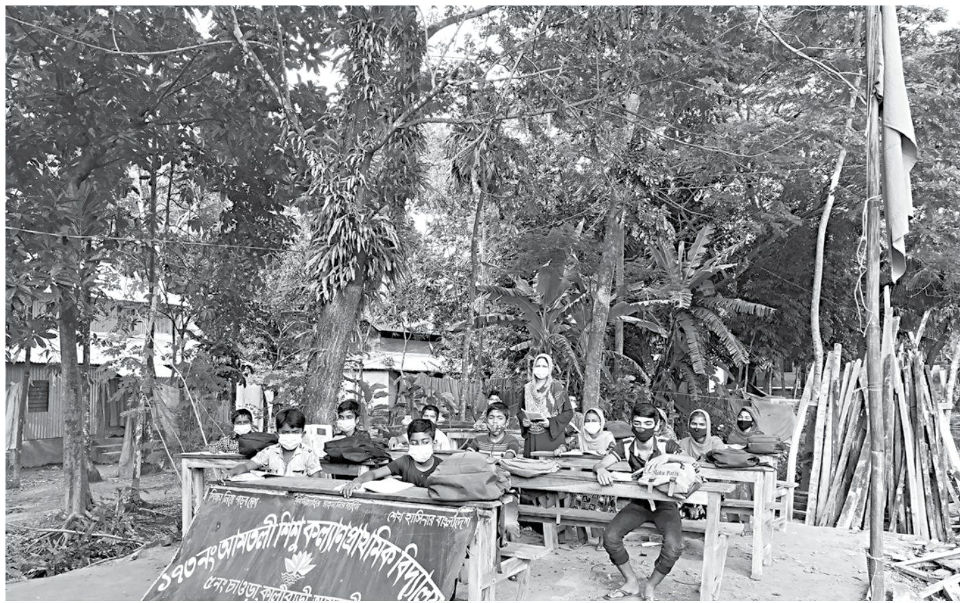
Students of Amtali Shishu Kalyan Primary School in Barguna's Amtali upazila attend classes under the open sky as their lone classroom collapses on Wednesday.
