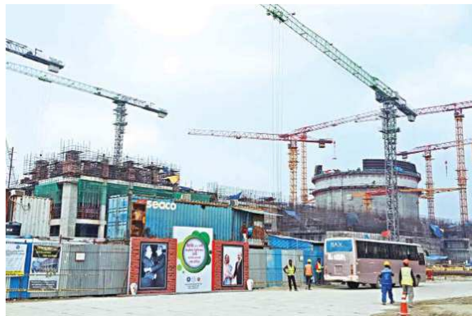
Of the Rooppur nuclear power plant's two units which would generate a combined 2,400 megawatts of electricity, the first (1,200MW) is expected to become operational from 2023 and the second in 2024. The photo was taken at the project site in Pabna's Ishwardi upazila yesterday.
