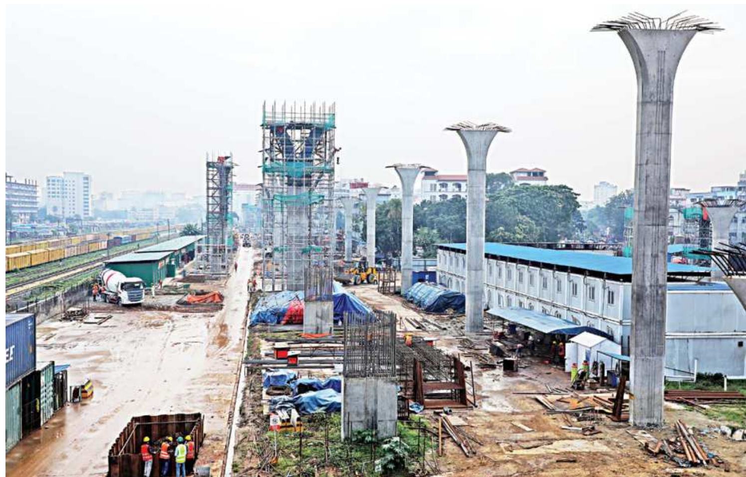
Construction work of Dhaka Elevated Expressway goes on in Tejgaon area yesterday. Road Transport and Bridges Minister Obaidul Quader last month said the whole project would be completed by June 2023. Once completed fully, the 19.73-kilometre expressway stretching from Hazrat Shahjalal International Airport to Kutubkhali on the Dhaka-Chattogram highway is expected to help people get across Dhaka without facing the huge traffic congestion within the city.
