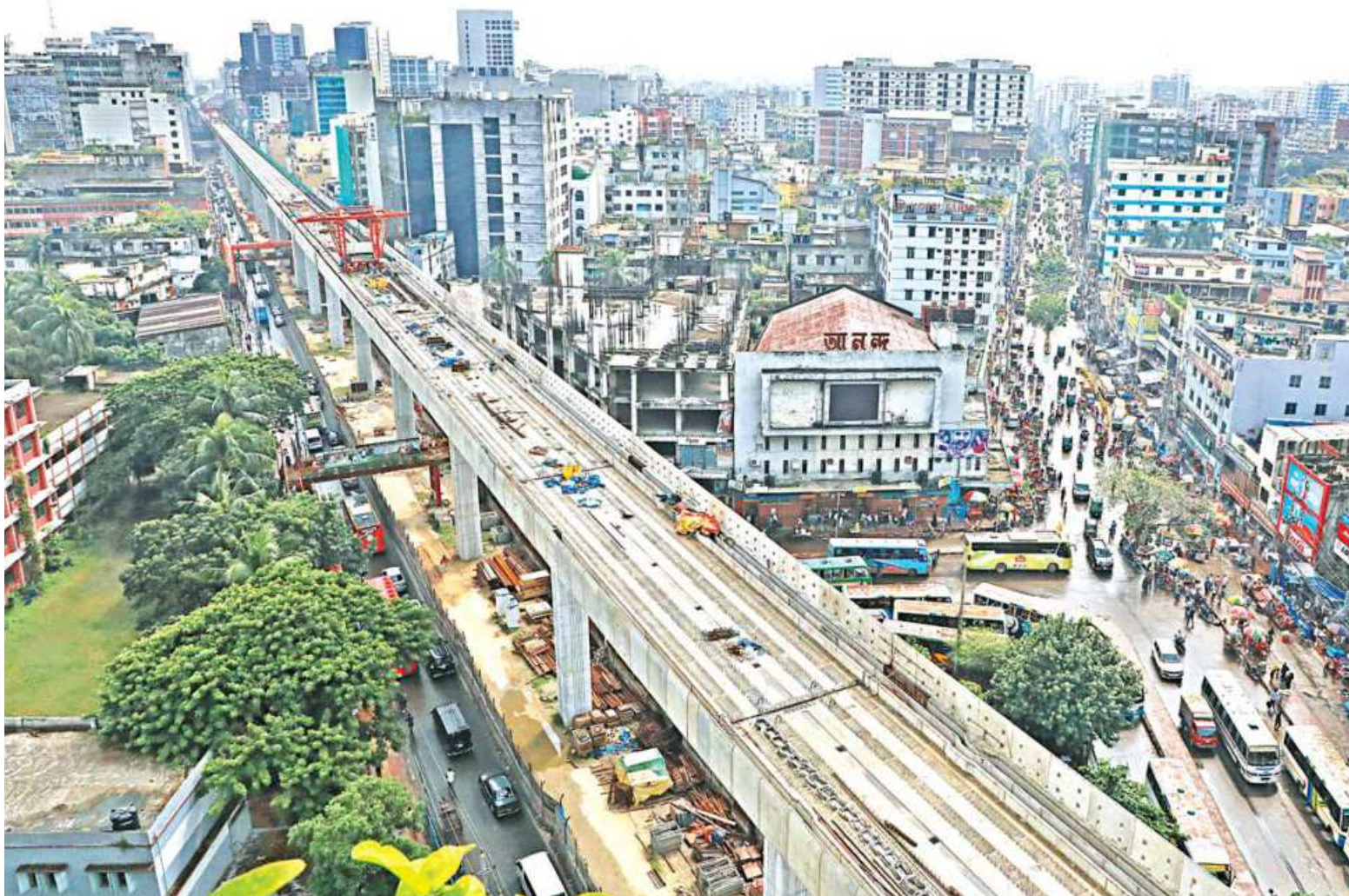
The Dhaka Mass Rapid Transit Development Project has seen physical progress of 50 per cent for its MRT-6 from Uttara Third Phase to Motijheel, with 73.04 per cent of its fund of Tk 21,985 crore having been spent. The photo was taken at Farmgate recently.
