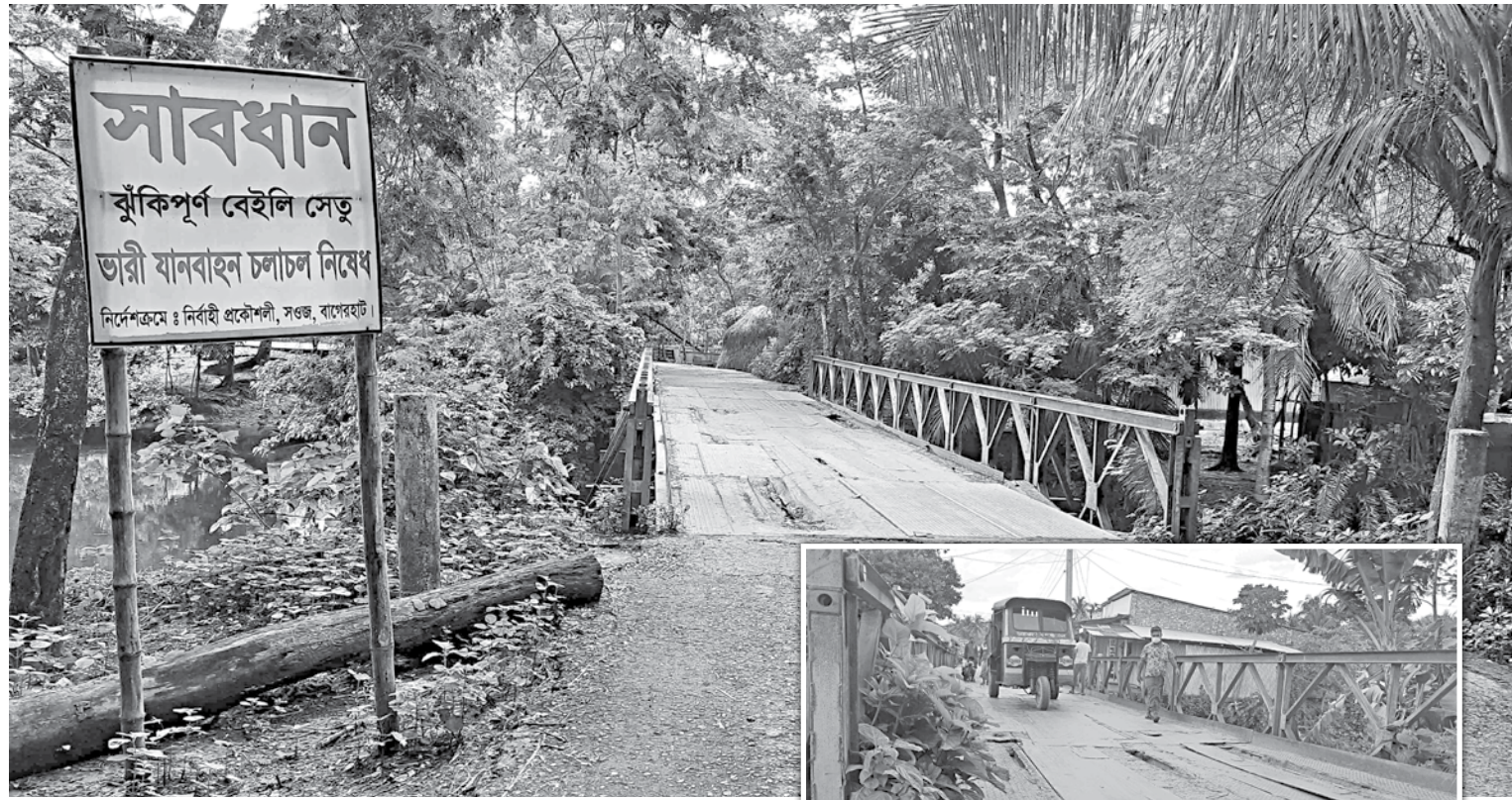
This two temporary bridges in Bagerhat's Mollahat upazila lie unrepaired for years, posing risk of accidents as well as disrupting vehicular movements.
