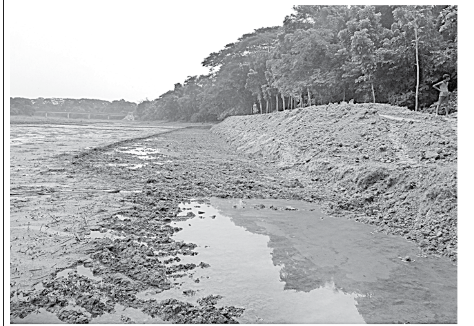
Kumar river's bank covering an area of 300 feet in length and 80 feet in width has been excavated by a local influential youth in Hatfadilpur bazar area under Shailakupa upazila of Jhenidah.
