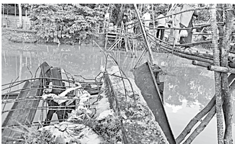
People built a bamboo bridge to cross Badura canal amid risk as the iron bridge over the waterbody in Pirojpur Sadar upazila has been lying broken for over seven years.
