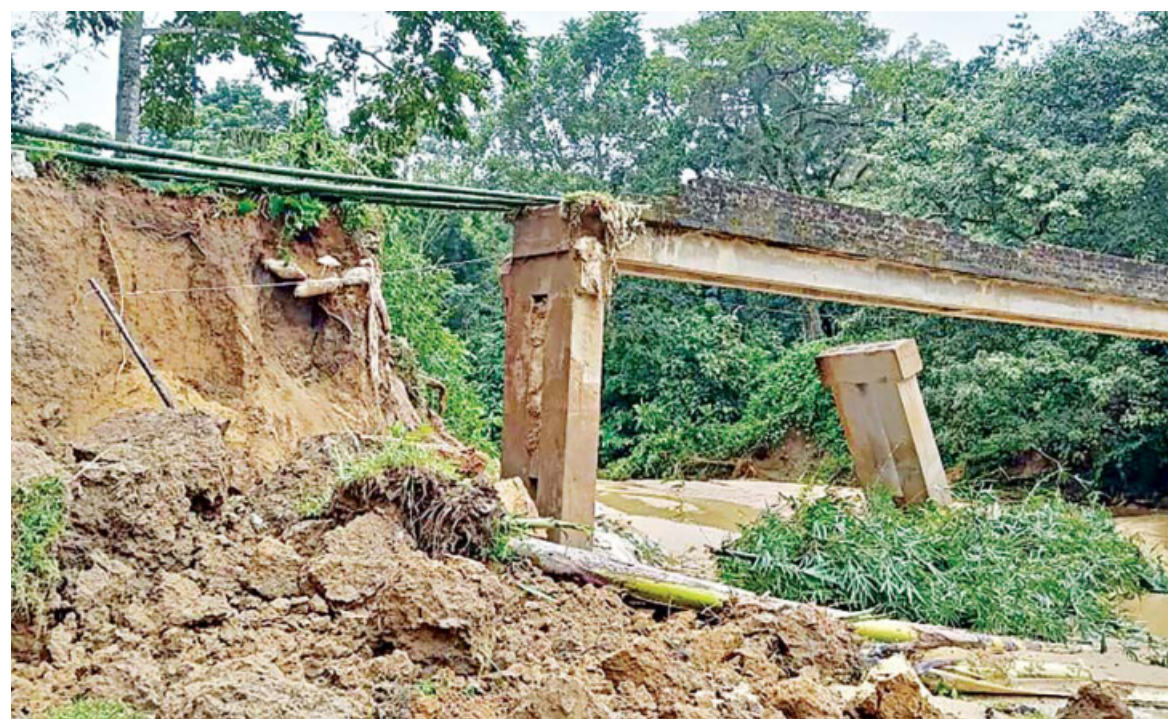
This partially collapsed and completely unusable bridge was the only way to a Tripura neighbourhood on a hill in Habiganj's Satchhari National Park. At least 20 Tripura families have not been able to leave their village since Wednesday, when the bridge fell amid heavy showers.
