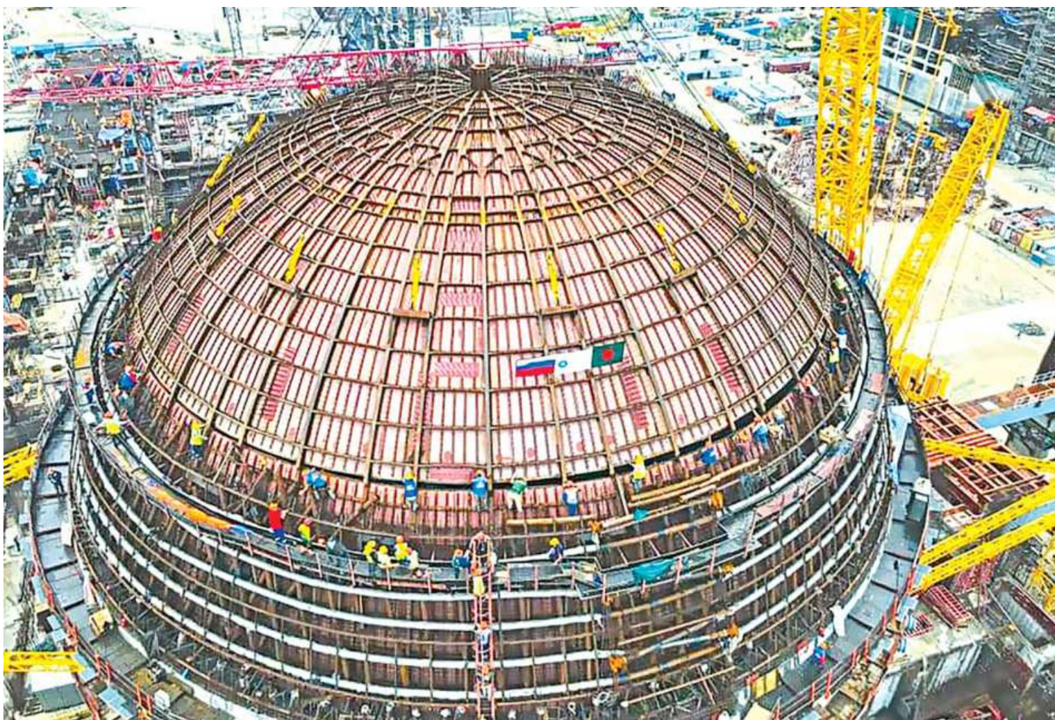
Construction work of a reactor in unit-1 of the Rooppur nuclear power plant is in progress. Prime Minister Sheikh Hasina will remotely inaugurate today the installation of the reactor pressure vessel at the power plant in Pabna. The pressure vessel is where electricity is generated from nuclear fuel, officials said.
