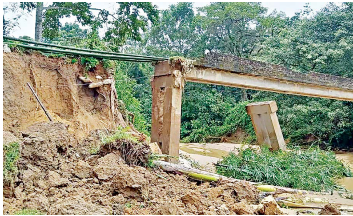
This partially collapsed and completely unusable bridge was the only way to a Tripura neighbourhood on a hill in Habiganj's Satchhari National Park. At least 20 Tripura families have not been able to leave their village since Wednesday, when the bridge fell amid heavy showers.
