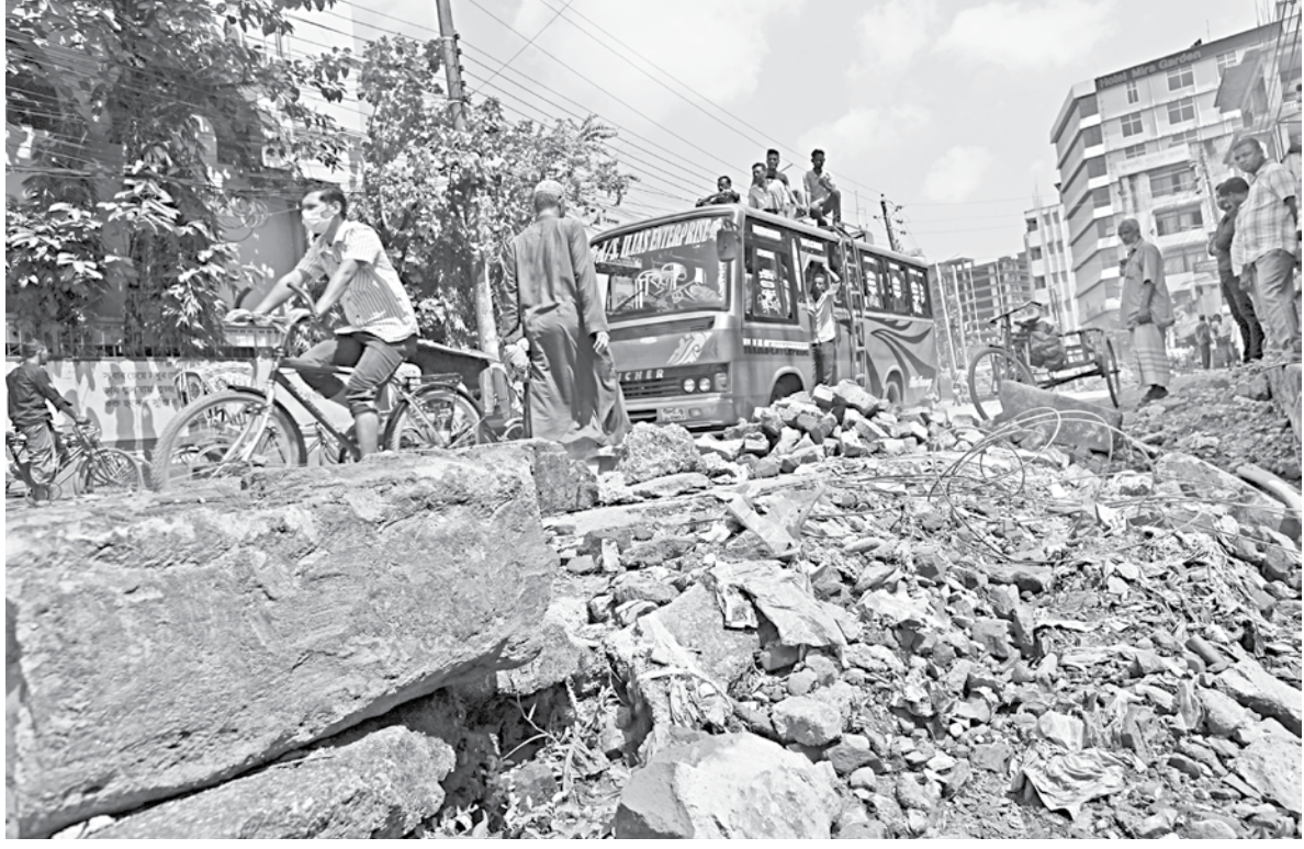
This broken section at Sylhet city's Nayorpu area is actually a drain that the city corporation has been working on for the last six months. With no signage to warn pedestrians and drivers, many get injured while traversing the debris. Locals say such negligence by authorities can lead to accidents and even loss of lives. This photo was taken yesterday.
