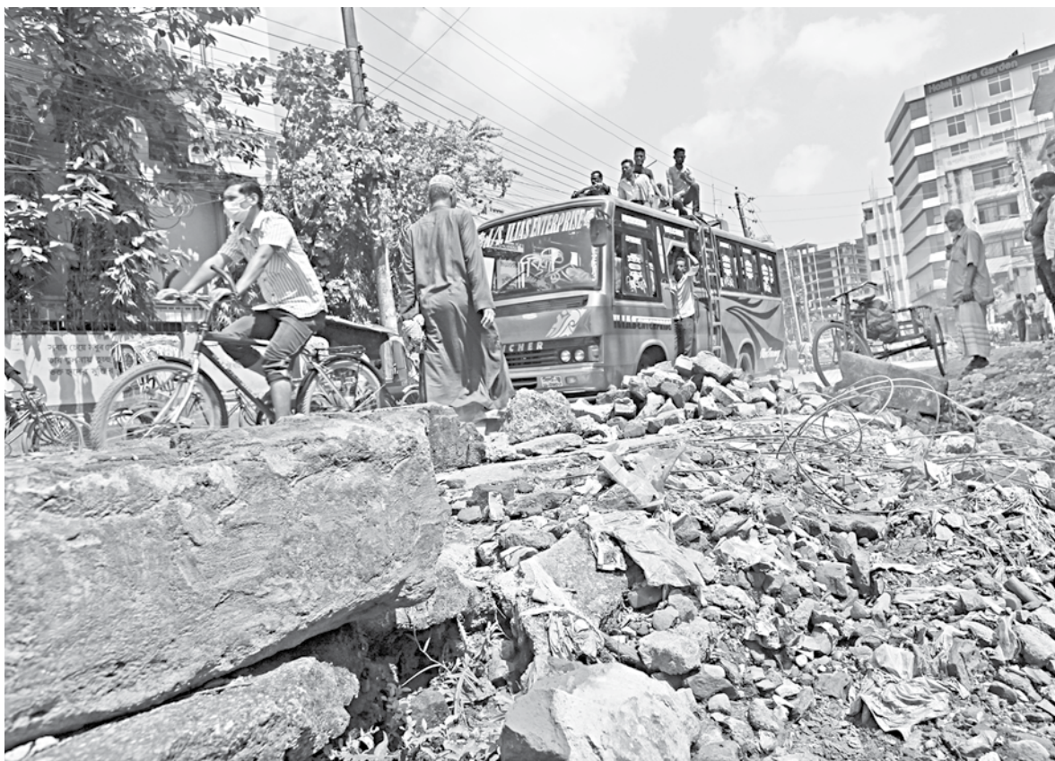
This broken section at Sylhet city's Nayorpu area is actually a drain that the city corporation has been working on for the last six months. With no signage to warn pedestrians and drivers, many get injured while traversing the debris. Locals say such negligence by authorities can lead to accidents and even loss of lives. This photo was taken yesterday.
