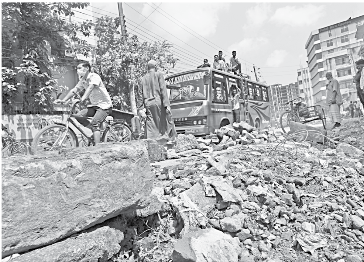
This broken section at Sylhet city's Nayorpu area is actually a drain that the city corporation has been working on for the last six months. With no signage to warn pedestrians and drivers, many get injured while traversing the debris. Locals say such negligence by authorities can lead to accidents and even loss of lives. This photo was taken yesterday.
