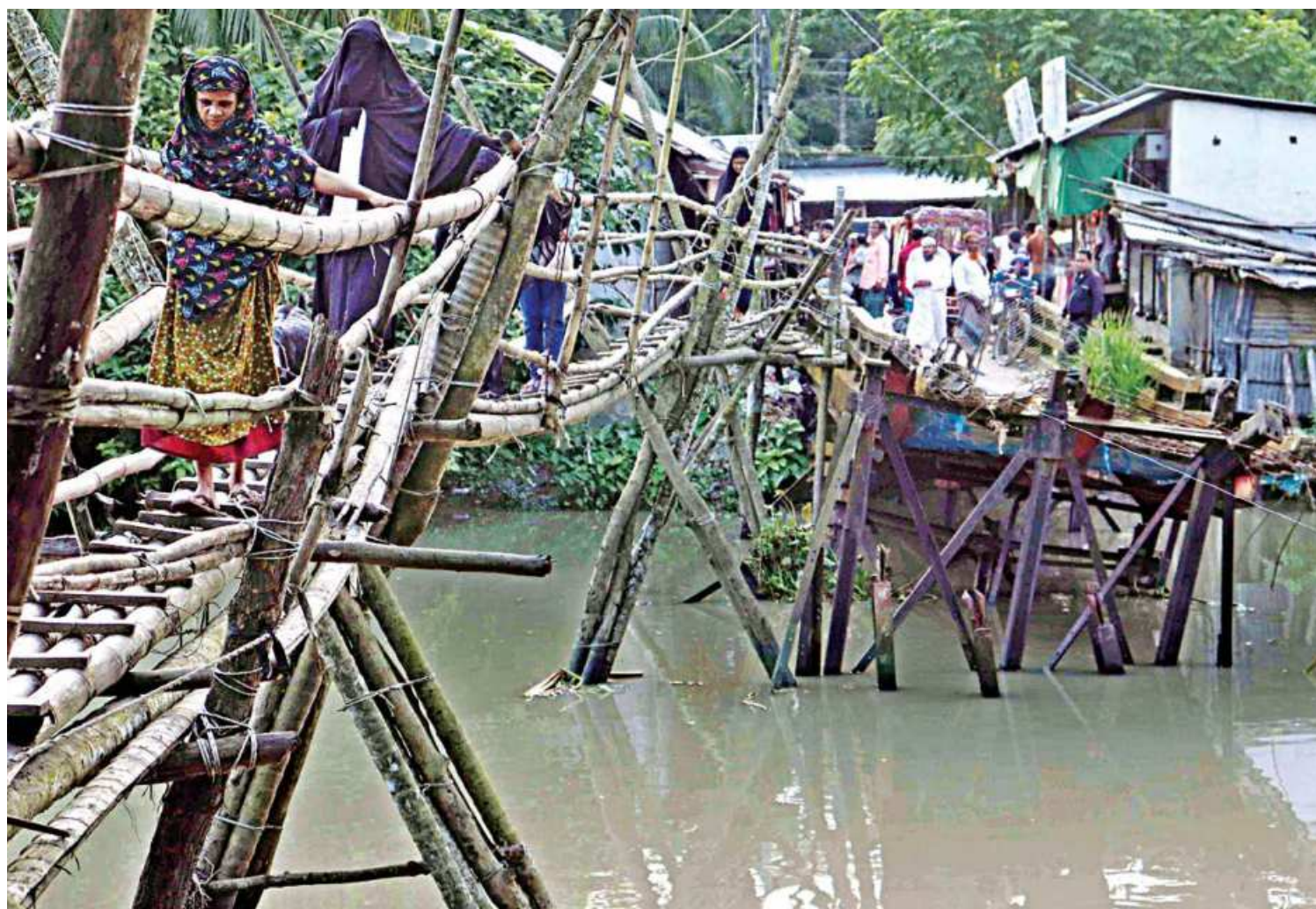
The iron bridge, on right of the photo, over the Badura canal near Mallik Bari Bus Stop in Pirojpur Sadar upazila has been in this sorry state for the last seven years. People built a bamboo bridge to cross the canal. Thousands of locals use this bridge with difficulty every day.
