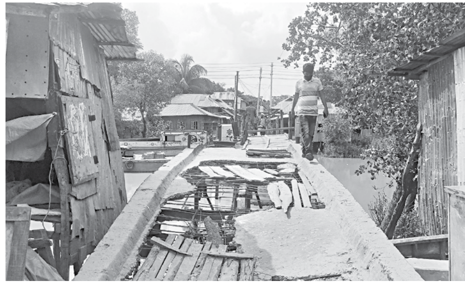
A man walks precariously on the edge of the bridge, on Gohinkhali canal in Patuakhali's Rangabali upazila, which was declared unfit by the LGED in 2012. However, the LGED is still awaiting approval for replacing this risky bridge with a new one.
