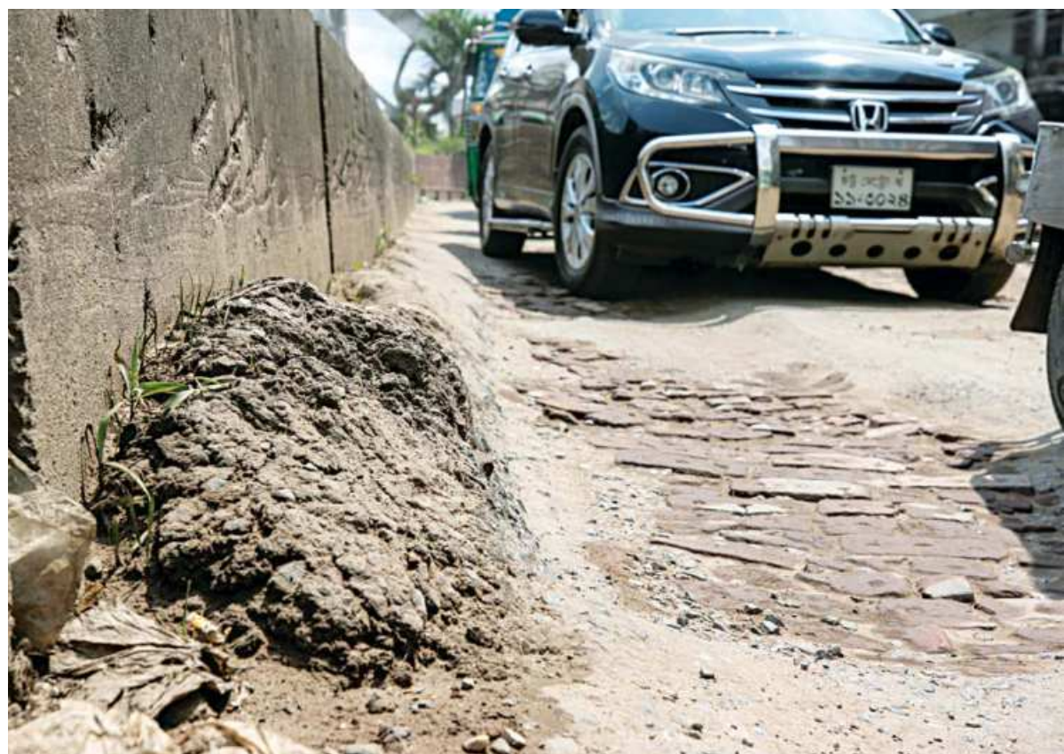
This road in the port city's Dewan Hat is in a bad state. Whether due to the use of low-quality construction material or regular use by large, overweight vehicles, the road has become synonymous with traffic tailbacks and frequent accidents in the Dhania Para area. This photo was taken yesterday.
