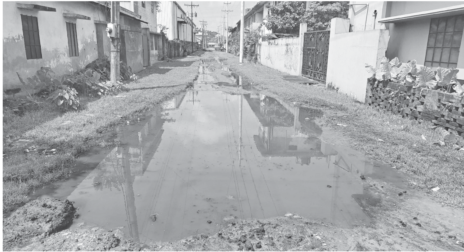
Lacking a proper drainage network and routine maintenance, pothole-riddled roads in Bagerhat BSCIC industrial area mostly look like this during the wet season.
