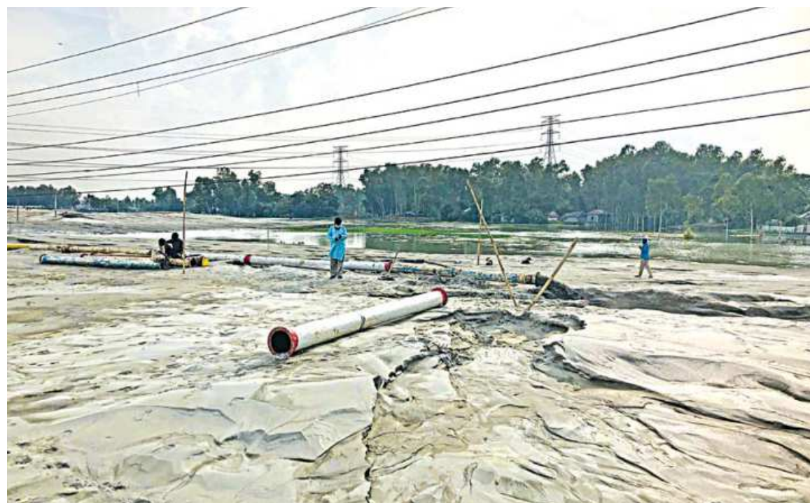
Earth-filling at the Sirajganj Economic Zone is underway. The country's largest private economic zone is expected to create five lakh jobs.
