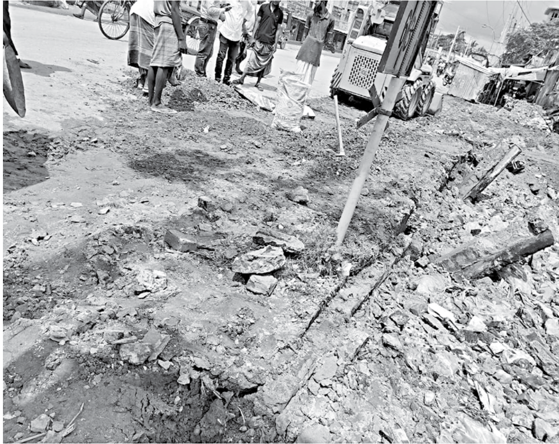
Workers using cement bags to remove rubble after a part of the wall belonging to BWDB was torn down in Kuakata town along Kuakata-Patuakhali highway. The photo was taken on September 25.
