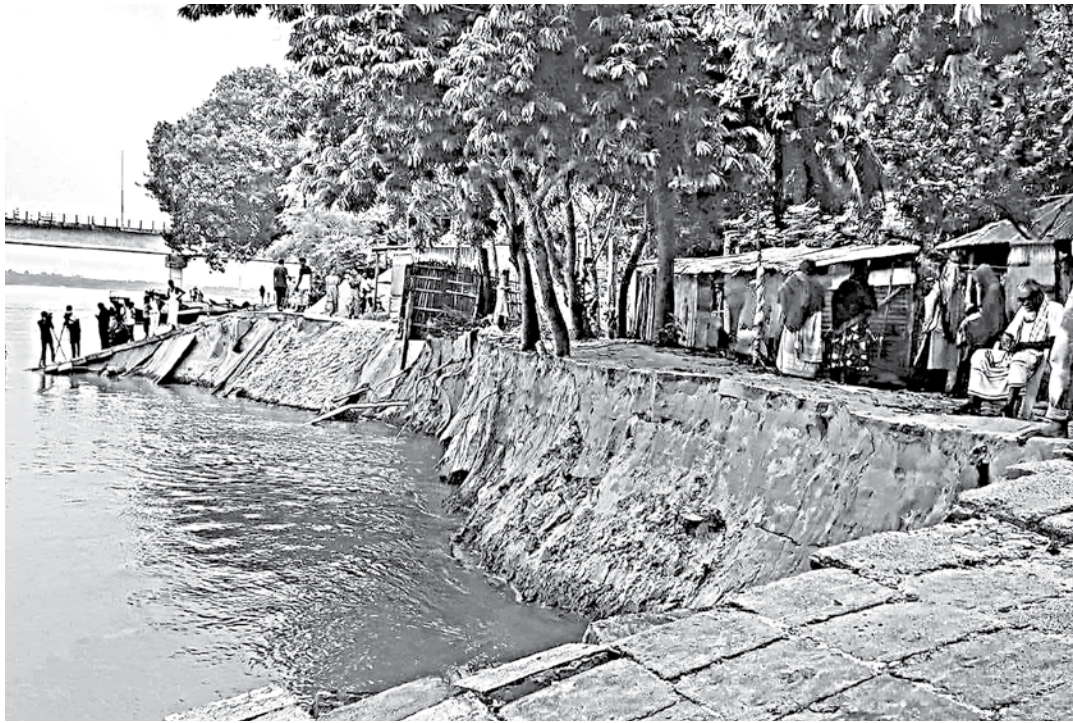
With the Sheikh Russell Bridge visible several hundred feet away, a large section of the bridge's protection embankment has eroded away by the Gorai river in Haripur union of Kushtia Sadar upazila. The photo was taken recently.
