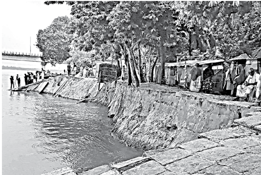
With the Sheikh Russell Bridge visible several hundred feet away, a large section of the bridge's protection embankment has eroded away by the Gorai river in Haripur union of Kushtia Sadar upazila. The photo was taken recently.
