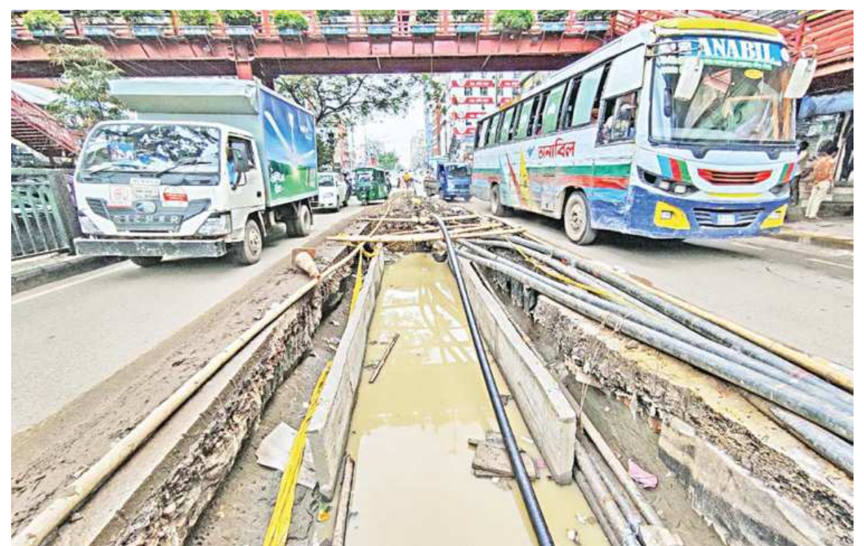
The DIC Road at the capital's Malibagh Chowdhury Para was dug right in the middle to install underground cables. A month on, the work is showing no signs of completion, piling an endless barrage of suffering on commuters. This photo was taken yesterday.
