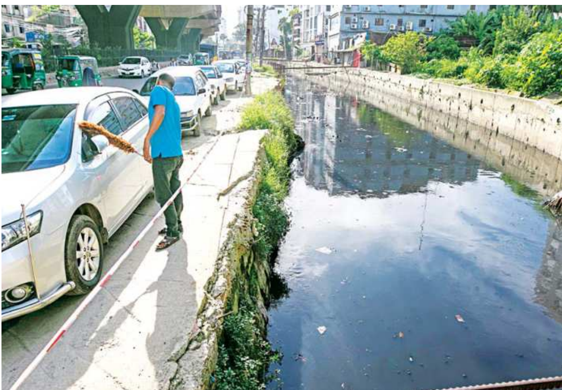
Only a flimsy tape protects this man, dusting the window of a car, from the wide open drain in Chattogram's Muradpur area. Many of the open drains in the port city do not even have that tape. Such open drains pose serious hazards for pedestrians. The photo was taken on Tuesday. PHOTO: RAJIB RAIHAN
