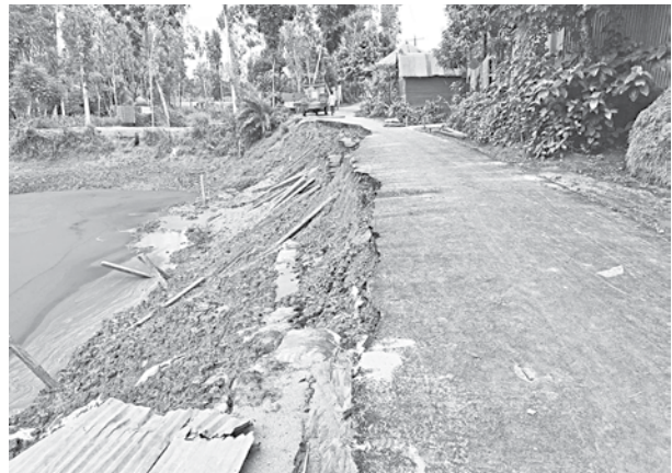
Portion of this newly built road at Ghargram village in Sirajganj's Tarash upazila collapsed in a roadside pond within 2 months of its construction.
