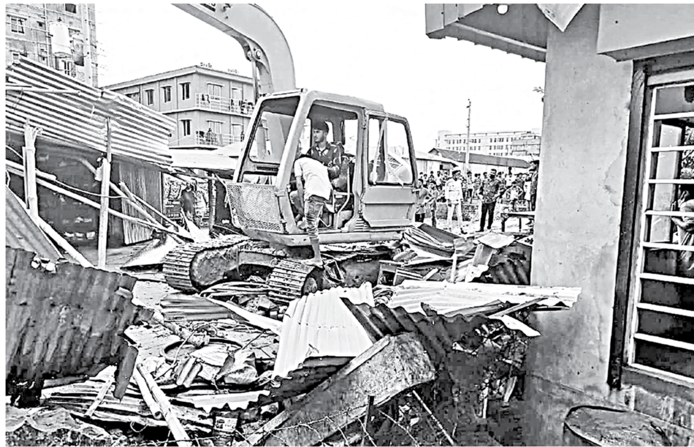
Blatantly disregarding law and court order, an excavator owned by the Gazipur City Corporation demolishes homes to make space for the city corporation's development projects. The photo was taken over a month ago.
