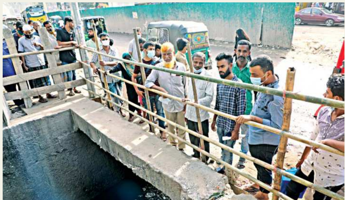
The tragic incident occurred at this drain in Agrabad's Badamtoli area. Unprotected the night before, when mild showers were sweeping across the city, the authorities have since propped up bamboo barriers around it yesterday.
