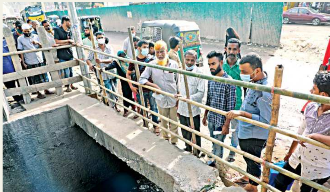
The tragic incident occurred at this drain in Agrabad's Badamtoli area. Unprotected the night before, when mild showers were sweeping across the city, the authorities have since propped up bamboo barriers around it yesterday.
