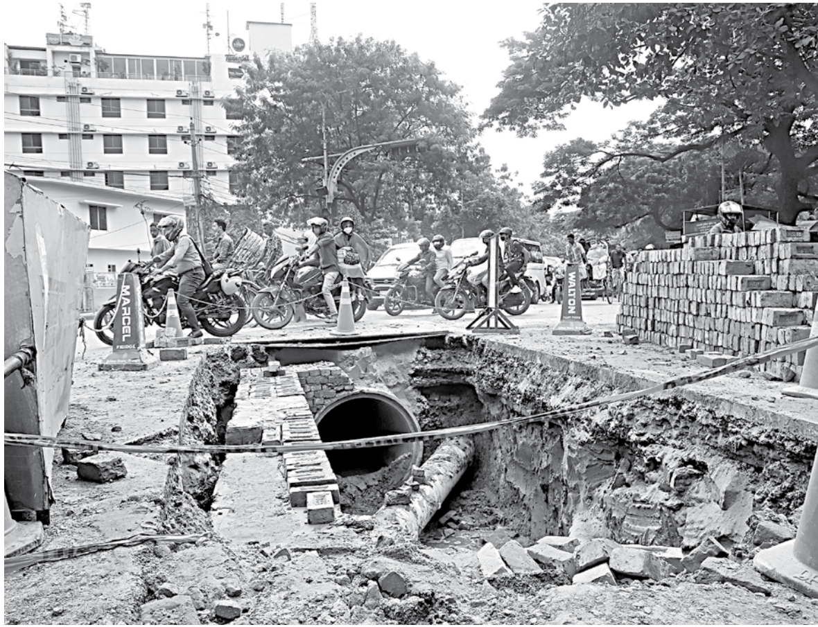
This has been the state of the Shahjahanpur intersection in the capital. For weeks, a part of the road has been cordoned off for Dhaka South City Corporation's development works, and commuters' suffering has reached an unbearable level as a result. This photo was taken yesterday.
