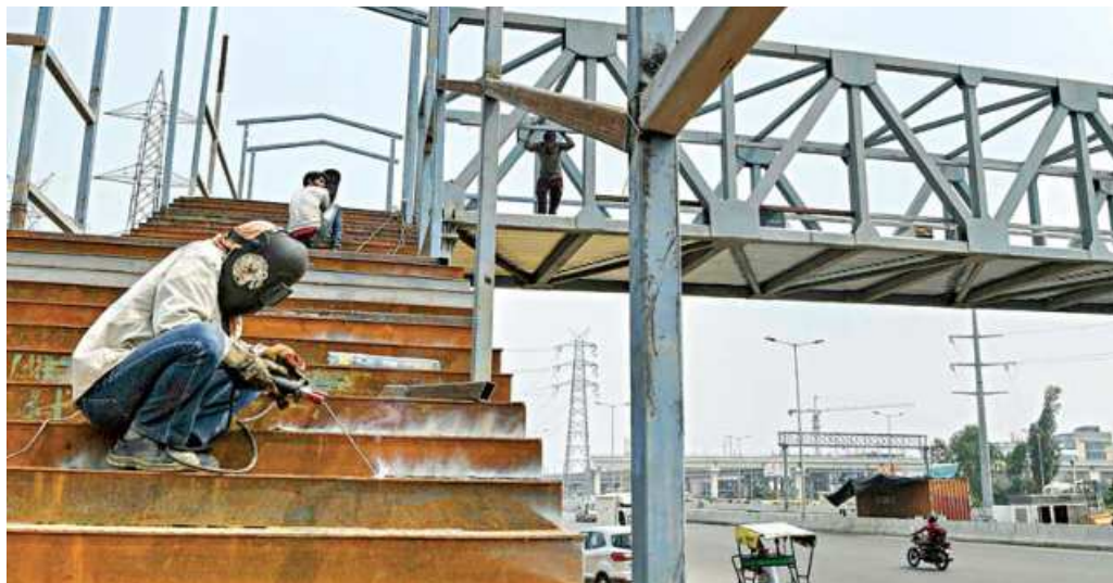
Workers build a bridge in Ghaziabad, India. The Asian Development Bank has cut its growth forecast for developing Asia.
