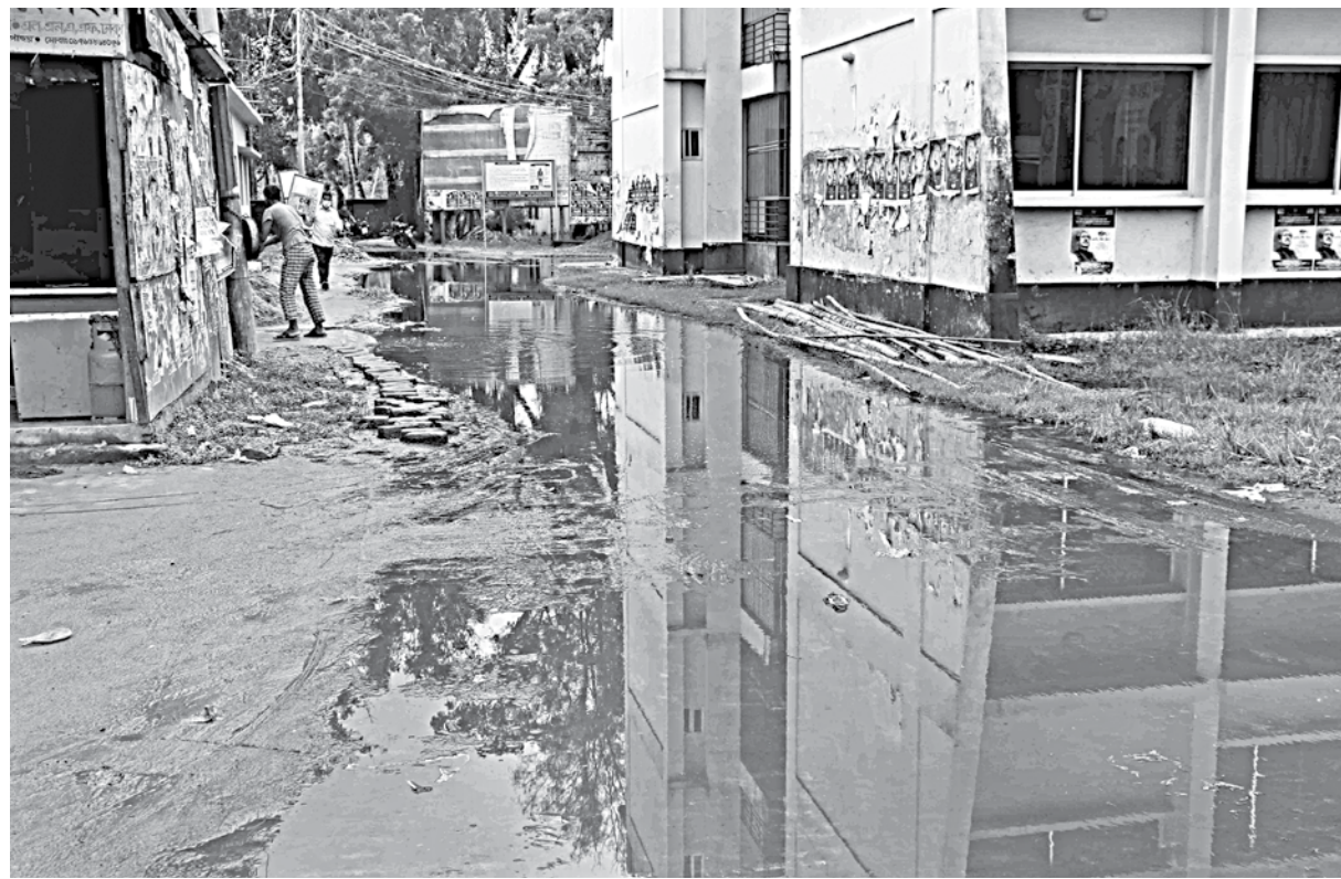
This important road to Pirojpur Sadar Upazila Parishad remains waterlogged for days even after a light rain, causing untold suffering to service seekers at different government offices. Locals blame unplanned construction of the road for the sufferings.
