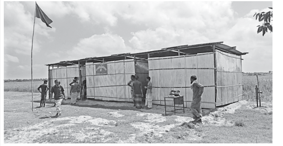
The temporary tin-roofed structure built for West Haldibari Government Primary School in Hatibandha upazila of Lalmonirhat.
