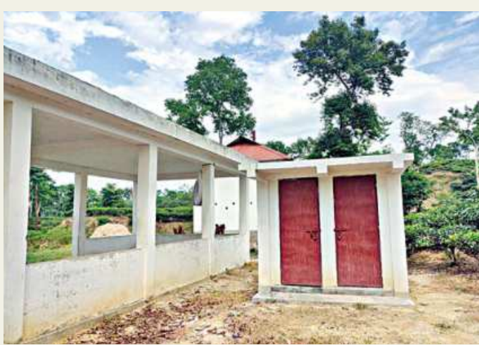
The two toilet facilities for tea garden workers at Mirzapore tea estate in Sreemangal.
