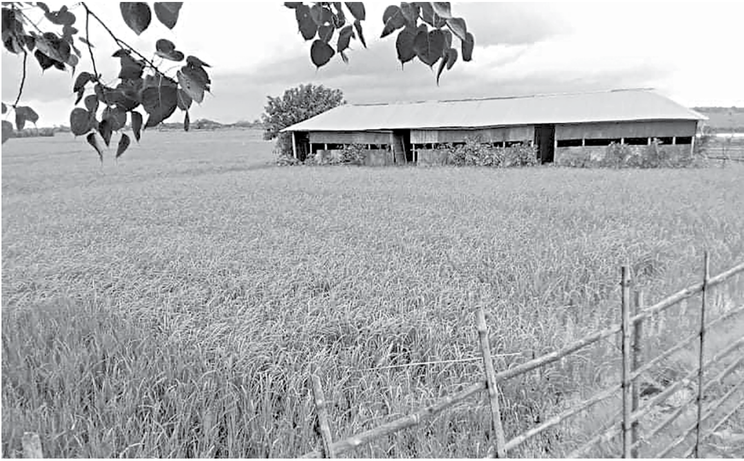
Ramnagar Poshchimpara Primary School in Kushtia's Mirpur upazila could not be reopened after Covid-19 restrictions were lifted recently, as rice cultivation in its playground has made the school inaccessible for all. PHOTO: AMANUR AMAN
