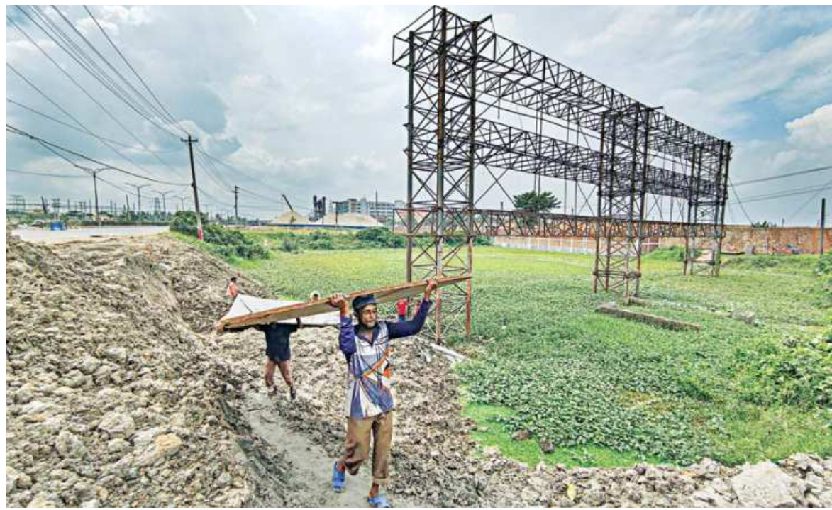
Workers dismantling a large hoarding from the side of the Dhaka-Aricha highway near Amin Bazar to make room for a new bridge there. After a bridge subsided disrupting traffic flow on the key highway, the authorities have decided to build the new structure with better capacity.
