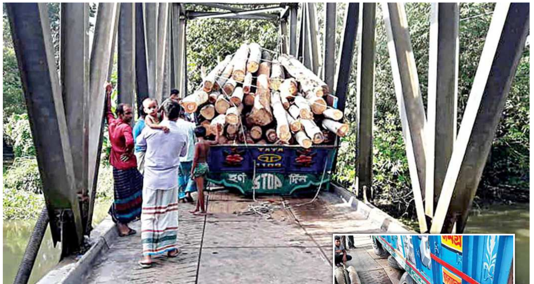
A timber-laden truck stuck on a Bailey bridge on the Tangail-Aricha regional highway in Tangail's Nagarpur upazila. Locals said a part of the surface of an already worn-out bridge was damaged when the truck was crossing it yesterday. Local administration officials said vehicles weighing more than eight tonnes were barred from using the bridge but that rule is flouted regularly. All 12 bridges on the regional highway are in varying stages of degradation.
