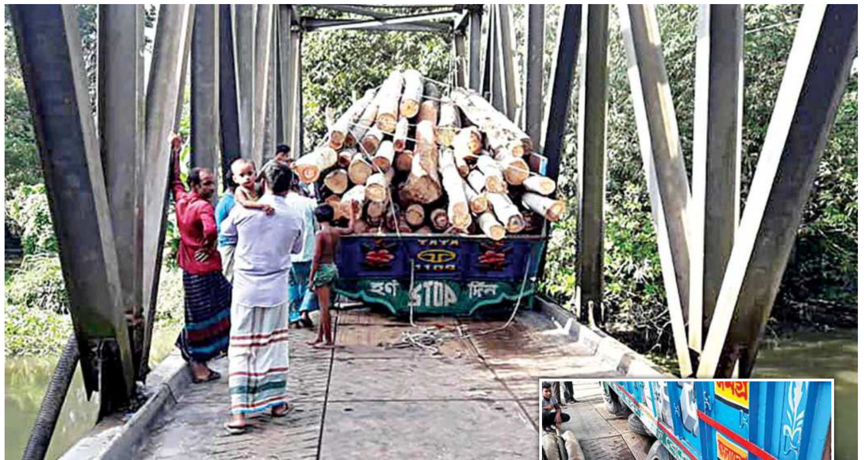
A timber-laden truck stuck on a Bailey bridge on the Tangail-Aricha regional highway in Tangail's Nagarpur upazila. Locals said a part of the surface of an already worn-out bridge was damaged when the truck was crossing it yesterday. Local administration officials said vehicles weighing more than eight tonnes were barred from using the bridge but that rule is flouted regularly. All 12 bridges on the regional highway are in varying stages of degradation.
