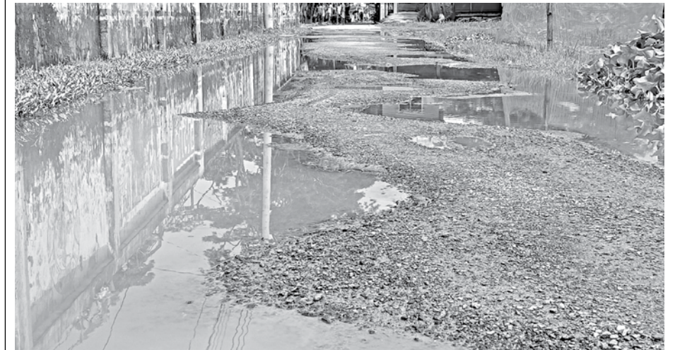
Part of a dilapidated road in Patuakhali's Kalapara town. The photo was taken recently.
