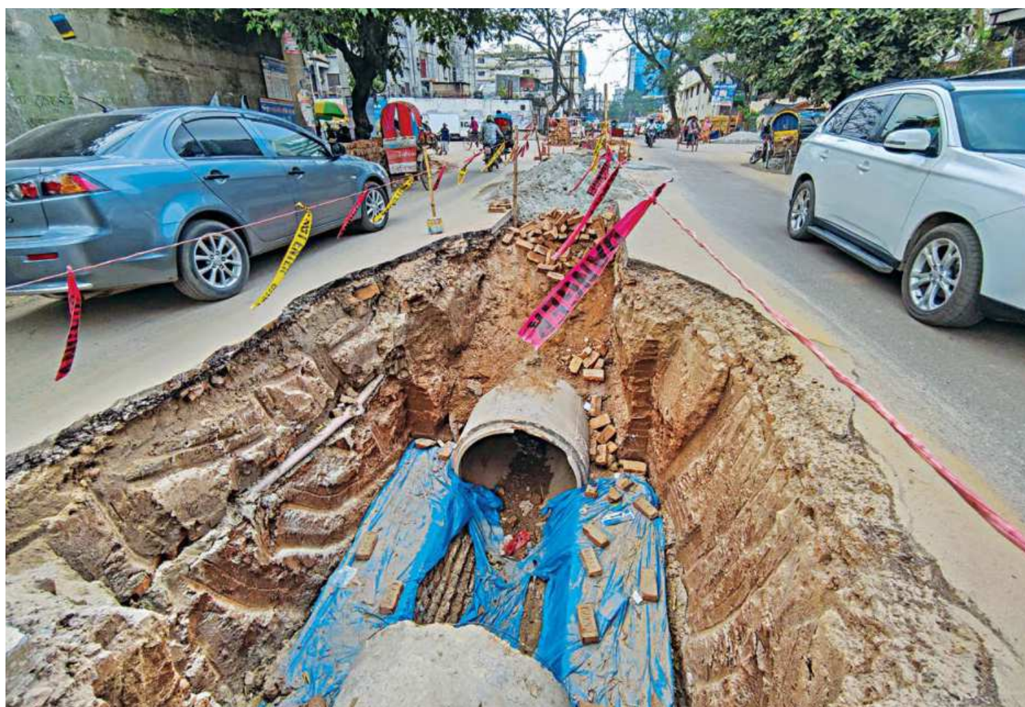
Without placing proper barriers, a large hole is dug right in the middle of a street near the capital's Tejgaon. Dhaka North City Corporation has dug such holes in several streets in Tejgaon for the installation of drainage pipes. Sometimes rainwater accumulates in these holes making it hard for motorists to realise the risk. The photo was taken yesterday.
