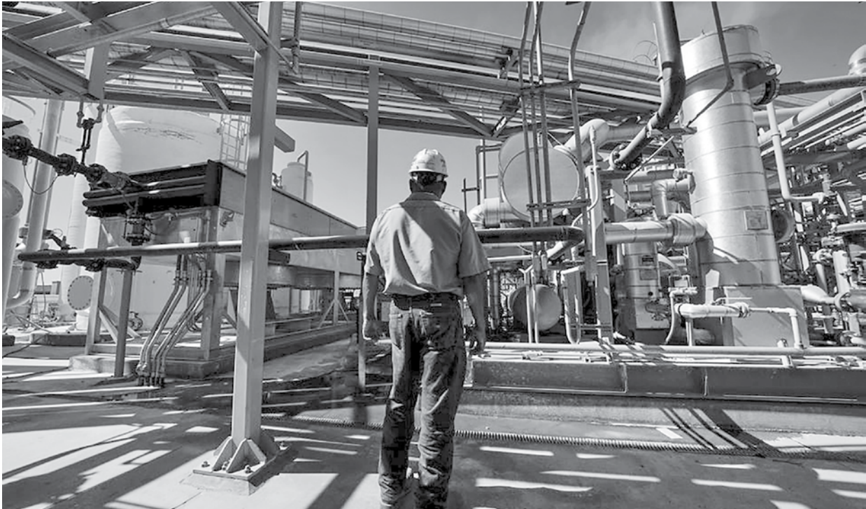
Calgren's renewable fuels facility that cleans dairy methane into natural gas is seen in Pixley, California, US.
