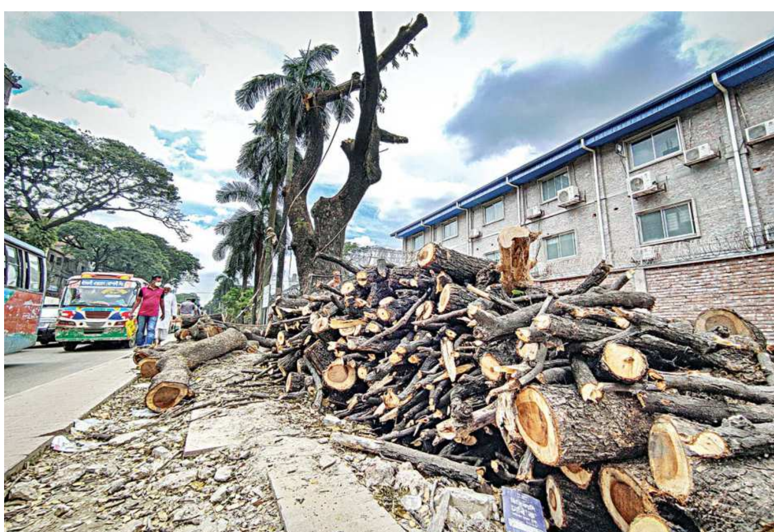
Many of the old trees on Indira Road between Farmgate intersection and Khamar Bari intersection have been chopped down for development work. The logs have been kept beside the pavement of the Sher-e-Bangla Nagar Park which is being used as a construction site for the metro rail project. The photo was taken yesterday. PHOTO: RASHED SHUMON
