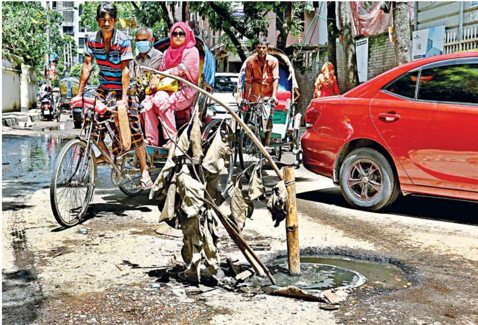
Near Baiy Road's Vqarunnisa Noon School and College campus, a manhole right down the middle of the 'tin rastar mor' is left uncovered. With no caution signs or barricades whatsoever, only a bamboo pole has been stuck inside it to warn pedestrians and vehicles of the danger it poses. Moreover, it's also become quite the nuisance for vehicular movement on the busy road that leads to the school and the nearby Monowara Hospital. The photo was taken yesterday.
