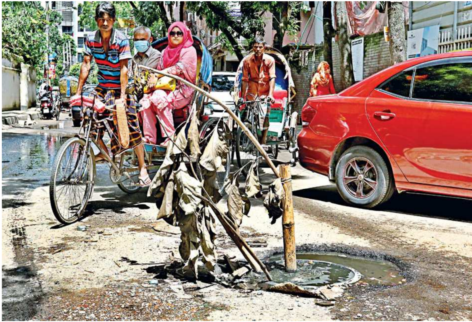
Near Baiy Road's Viqarunnisa Noon School and College campus, a manhole right down the middle of the 'tin rasta mor' is left uncovered. With no caution signs or barricades whatsoever, only a bamboo pole has been stuck inside it to warn pedestrians and vehicles of the danger it poses. Moreover, it's also become quite the nuisance for vehicular movement on the busy road that leads to the school and the nearby Monowara Hospital. The photo was taken yesterday.
