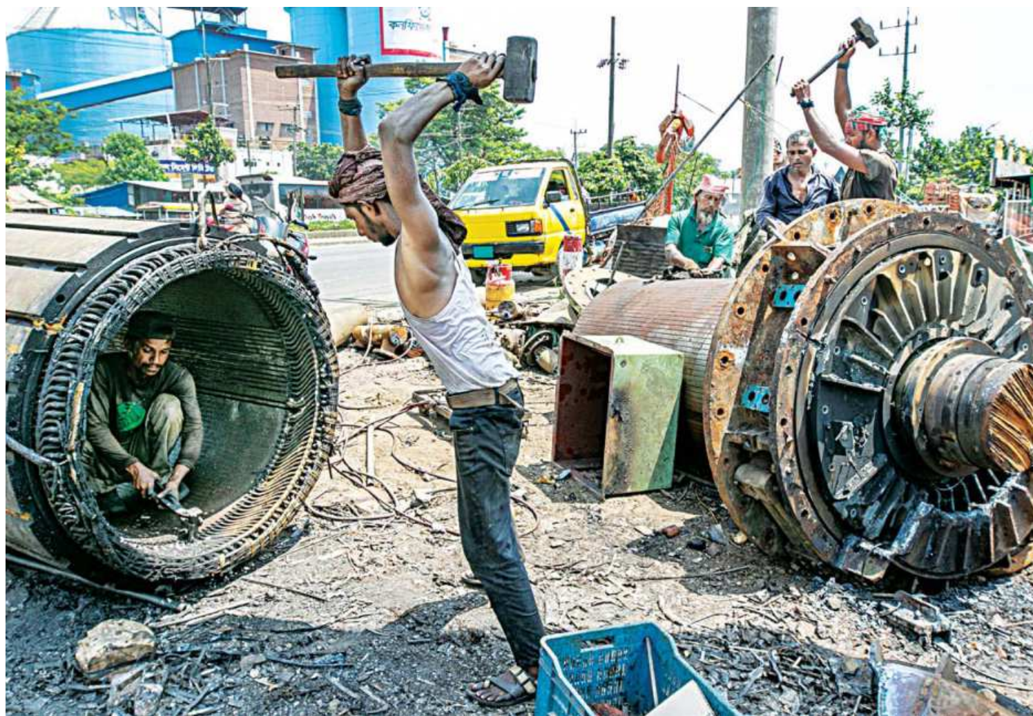
Large motors of old ships are being dismantled to extract valuable metals, including iron and copper. This photo was taken from Bhatiari of Chattogram's Sitakunda recently.
