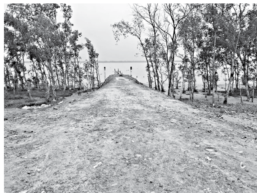
The under-construction ramp of the Rayenda ferry terminal on the bank of the Baleshwar river in Sharankhola upazila of Bagerhat. PHOTO: COLLECTED
