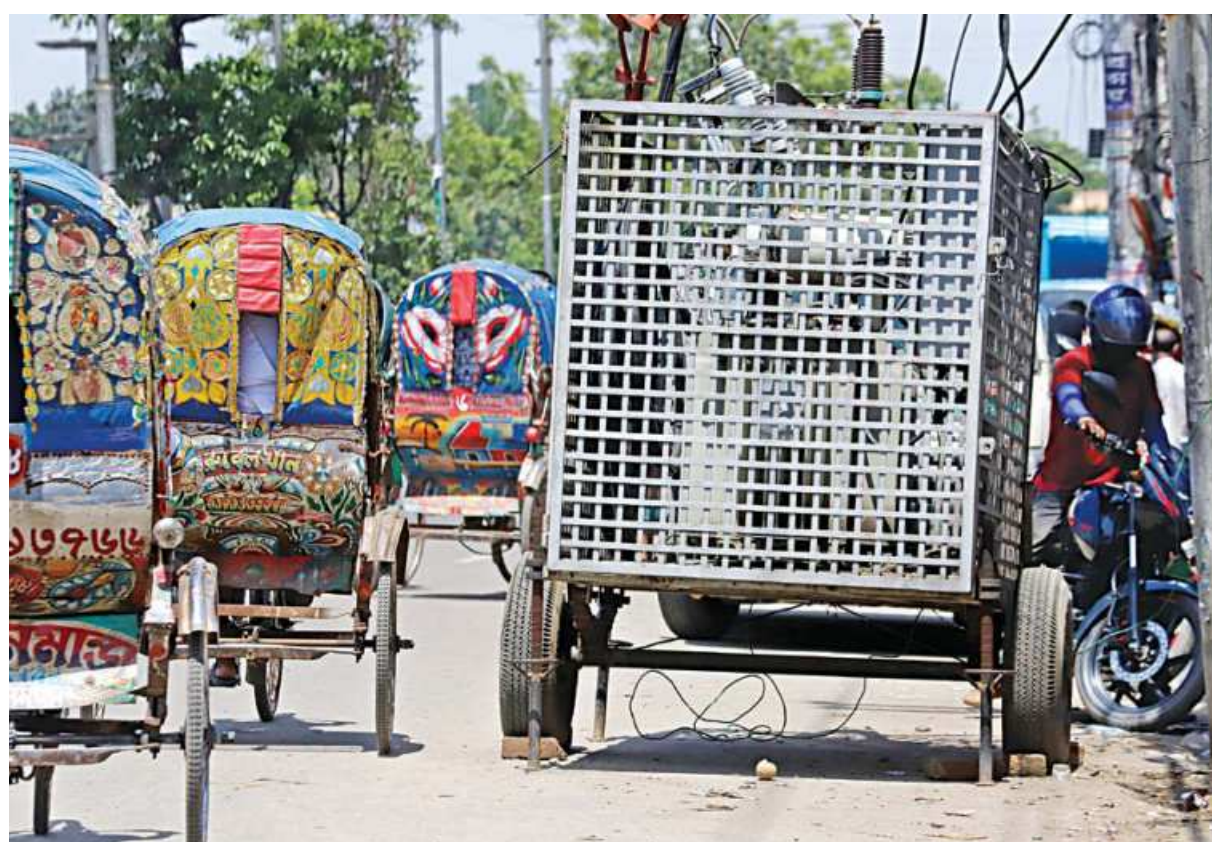
A mobile transformer has been left parked at Mugdapara's CNG Station area in the capital. Not only is it obstructing traffic on the busy road, but also posing electrocution risk for commuters of the area. This photo was taken yesterday.
