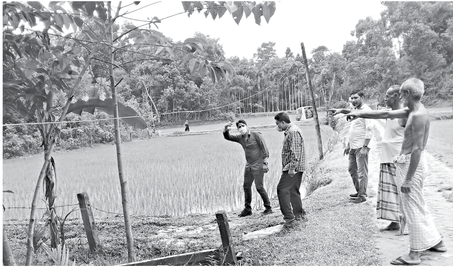
In this recent photo taken in Putadaha village of Moulvibazar's Barlekha upazila, villagers show the un-insulated single-phase live electrical wire dangling right above their heads.
