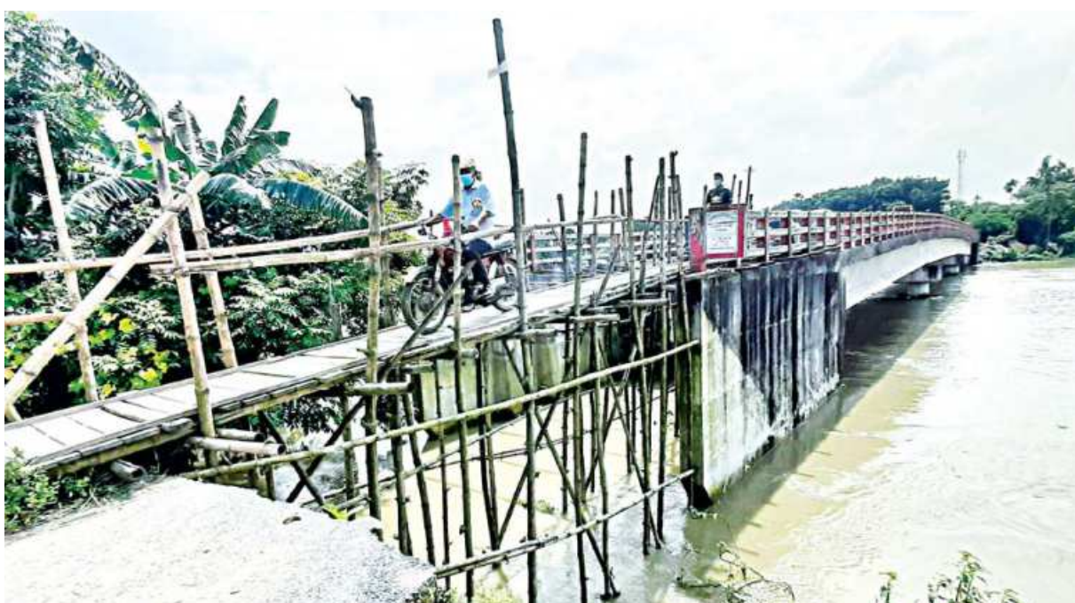
Locals in Tangail Sadar upazila's Boro Basalia area have been suffering for 14 long months as the mouth of a bridge over the Louhajang river remains damaged. The bridge leads to a road, which is important for communication in the upazila.
