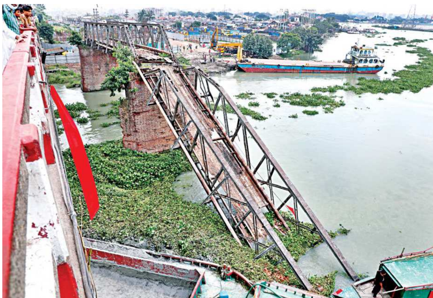
Part of the old iron Bailey Bridge in the capital's Aminbazar has collapsed into the river. Locals have alleged that the collapse occurred after a sand-laden trawler hit one of its pillars. There are other such collapsed structures around the bridge, and those could lead to further accidents if not cleared soon.
